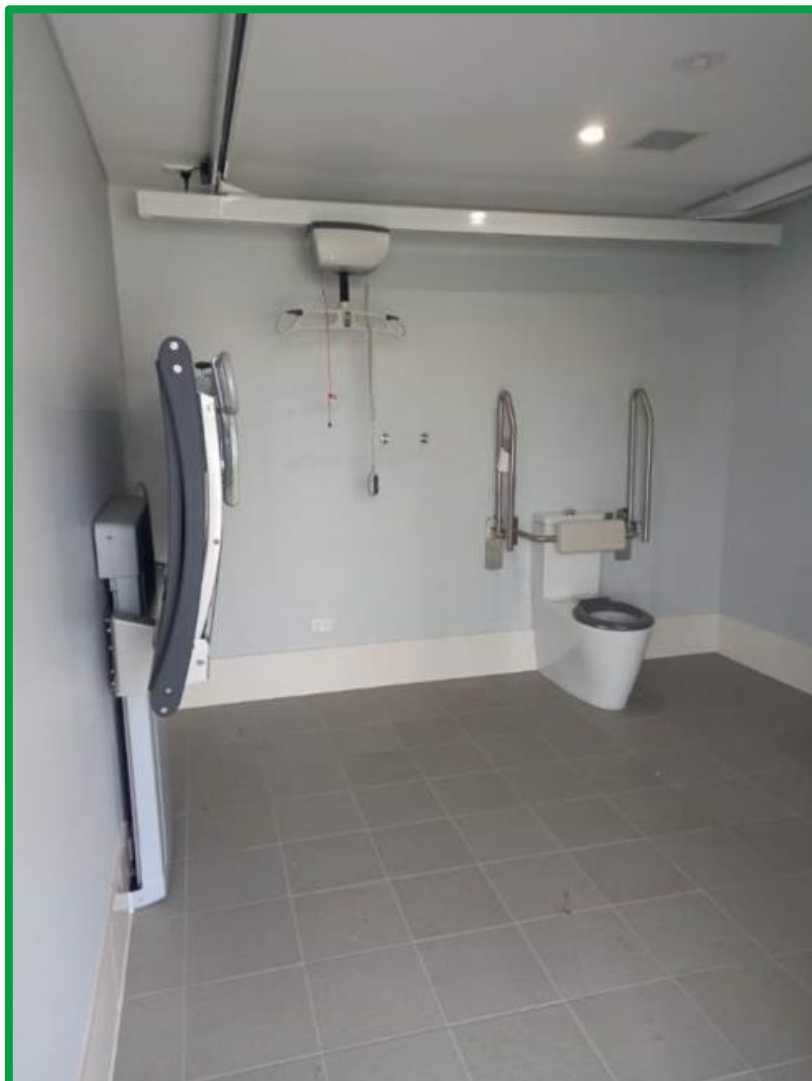
New crane lift in accessible toilet at Warren War Memorial Swimming Pool
